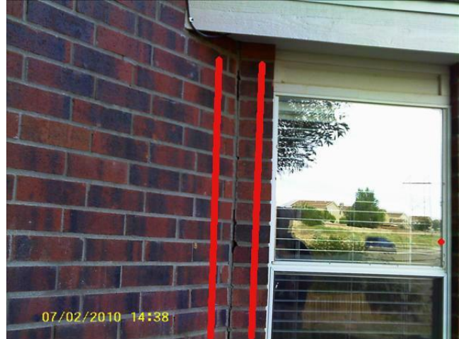
Exterior Structure Siding Condition Maintenance
