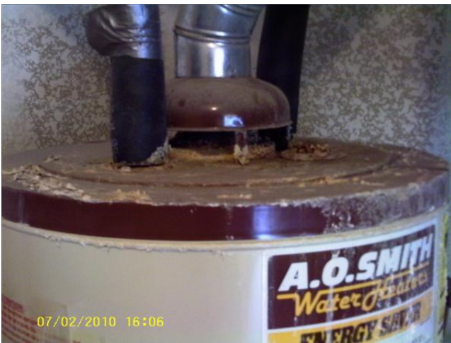
Water Heater Evidence of Encrustation Yes
