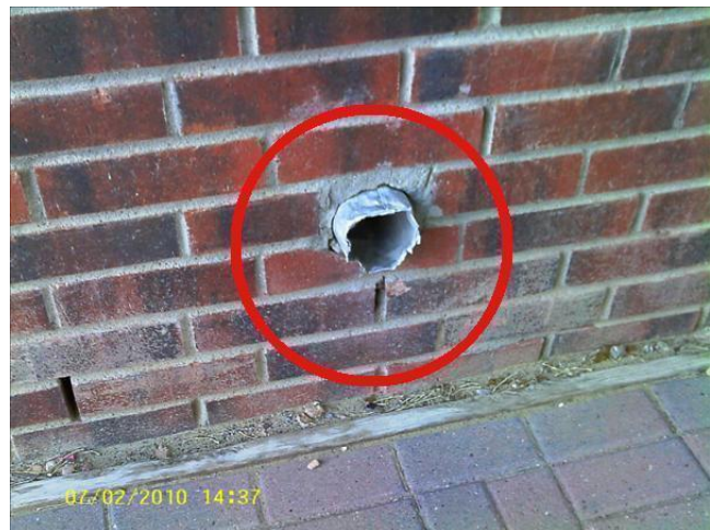
Laundry Area Dryer Ventilation System Attention
