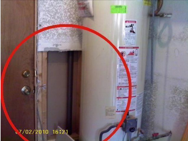
Attached Garage Fire Wall/Ceiling Board Action Required
