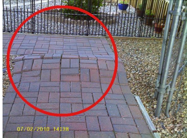
Site Concrete and Paving Walkways Attention
