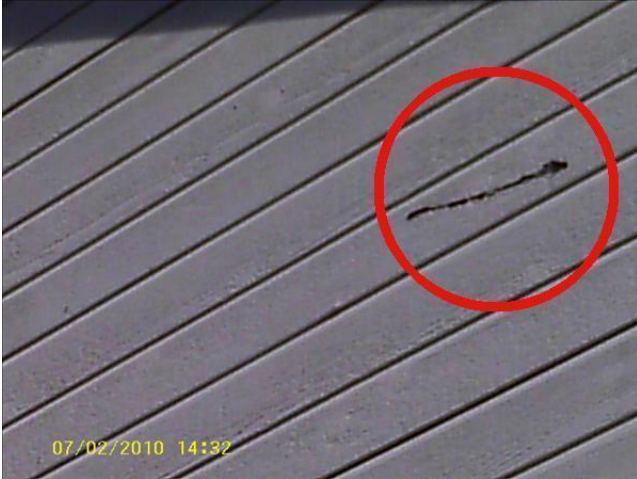
Exterior Structure Siding Condition Maintenance
